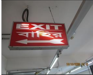
Photo of fire safety equipment Electric exit sign.JPG
