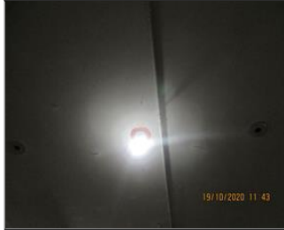
Photo of fire safety equipment Emergency light.JPG
