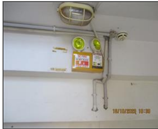
Photo of fire safety equipment Industrial graded emergency light.JPG
