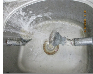
Photo of the inside of the main production hall Eye wash station.JPG
