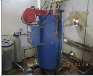
External photo(s) of the production unit(s) Boiler room.JPG
