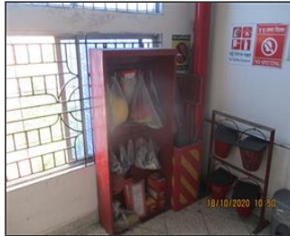
Photo of fire safety equipment Firefighting equipment.JPG
