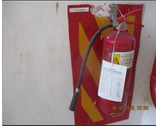
Photo of fire safety equipment Fire extinguisher.JPG
