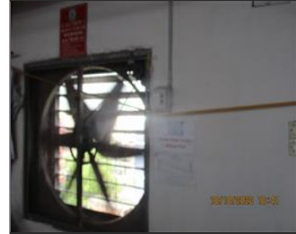
Photo of the inside of the main production hall Exhaust fan with safety instructions.JPG
