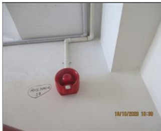
Photo of fire safety equipment Fire alarm.JPG
