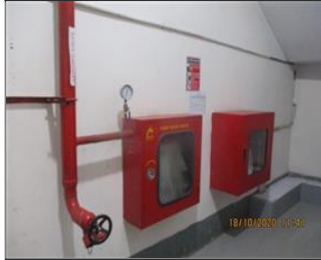
Photo of fire safety equipment Fire hose reel pipe.JPG
