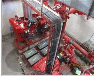
Photo of fire safety equipment Wet riser system.JPG
