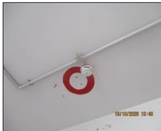
Photo of fire safety equipment Smoke detector.JPG
